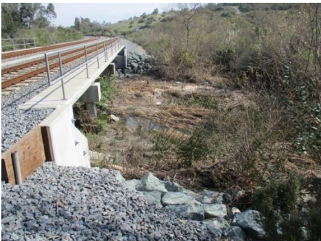
The Loma Alta Creek crossing onto the subject property near the center of the north subject property border looking east.
